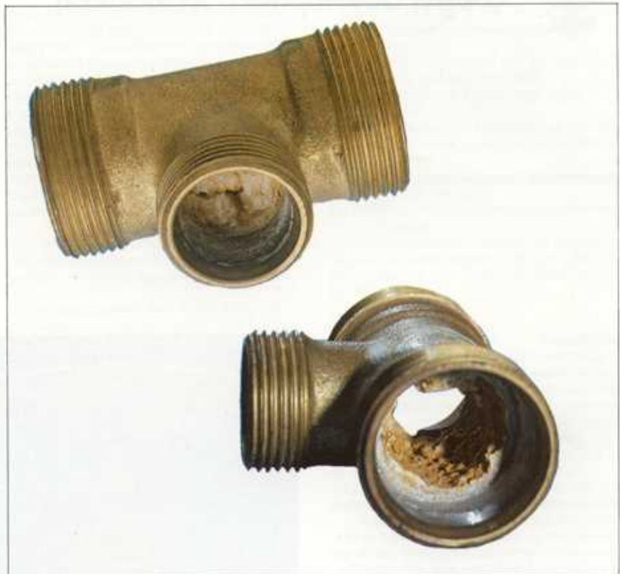
A duplex brass fitting showing the soft, white 'meringue' corrosion product basic zinc carbonate, which is severely restricting water flow.
