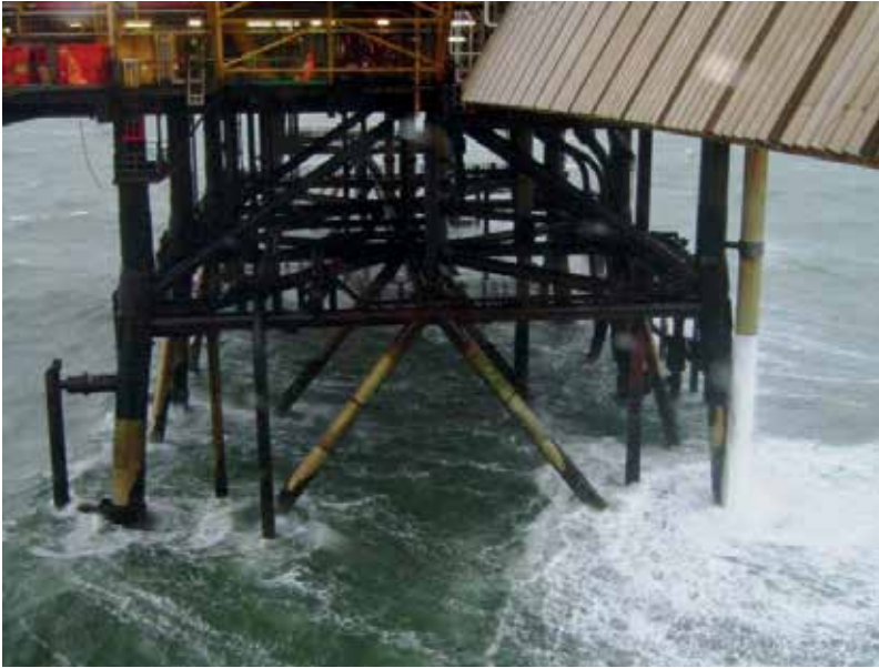
90-10 copper-nickel splash zone protection on a platform in the Morecambe Field, UK. The sheathing has been in service over 25 years (Courtesy Centrica Energy Upstream, East Irish Sea)
