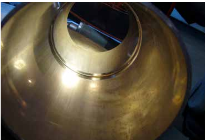
Finished weld showing root penetration on pipe bore (Courtesy Eucaro Buntmetall GmbH)
