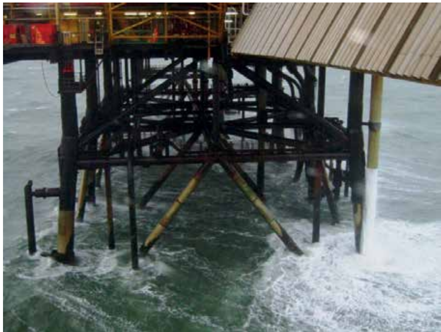
Figure 13 – 90-10 copper-nickel splash zone protection on a platform in the Morecambe Field, UK (Courtesy Centrica Energy Upstream, East Irish Sea)
