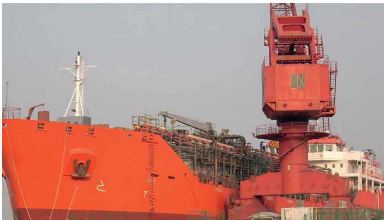
Figure 2 - Copper-nickel pipework aboard ship (Courtesy Eucaro Buntmetall GmbH)
